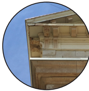
Damaged Soffit, Sheet Metal
