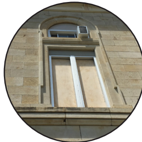
Infill Panels at Windows; Lack of Weather Barrier
