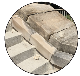
Deterioration at Limestone Masonry
